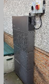
...and a 15kw battery to take advantage of cheap overnight Electricity in the winter when the sun dosen't shine!
